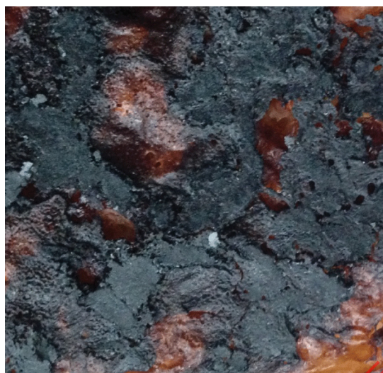
Figure C.13 – Example of Level 13 of burnt condition
